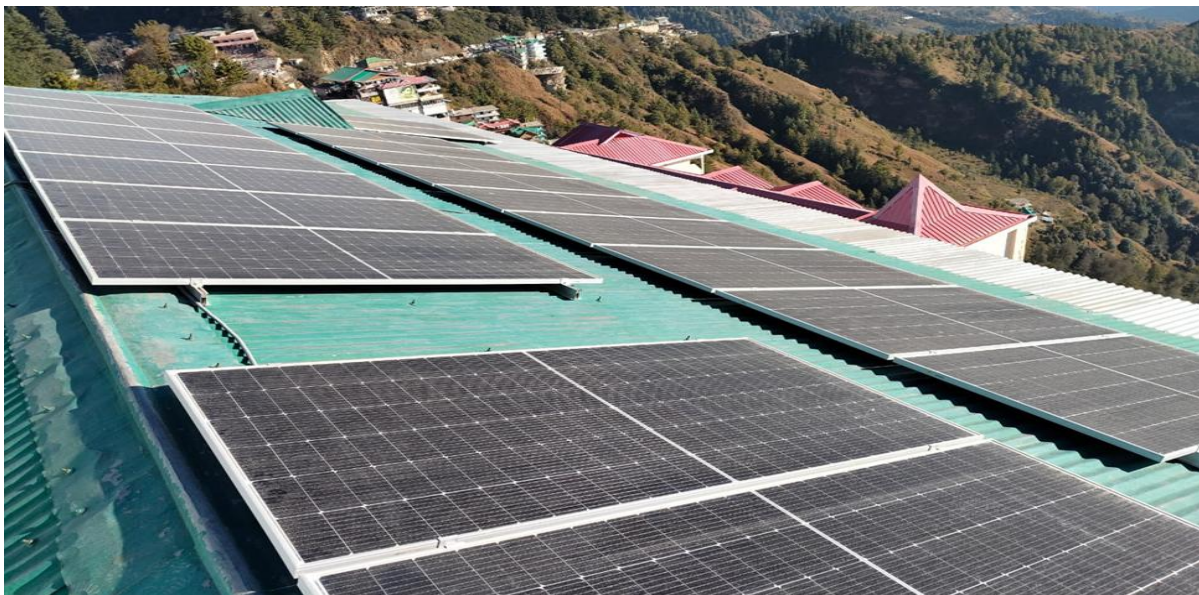
Solar Panel installed on College Building rooftop by Himurja
