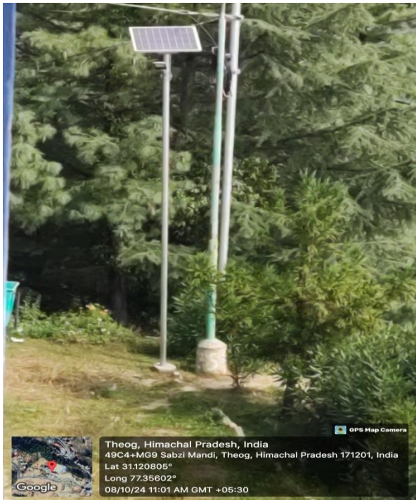
Solar Light (Backside of College Building)
