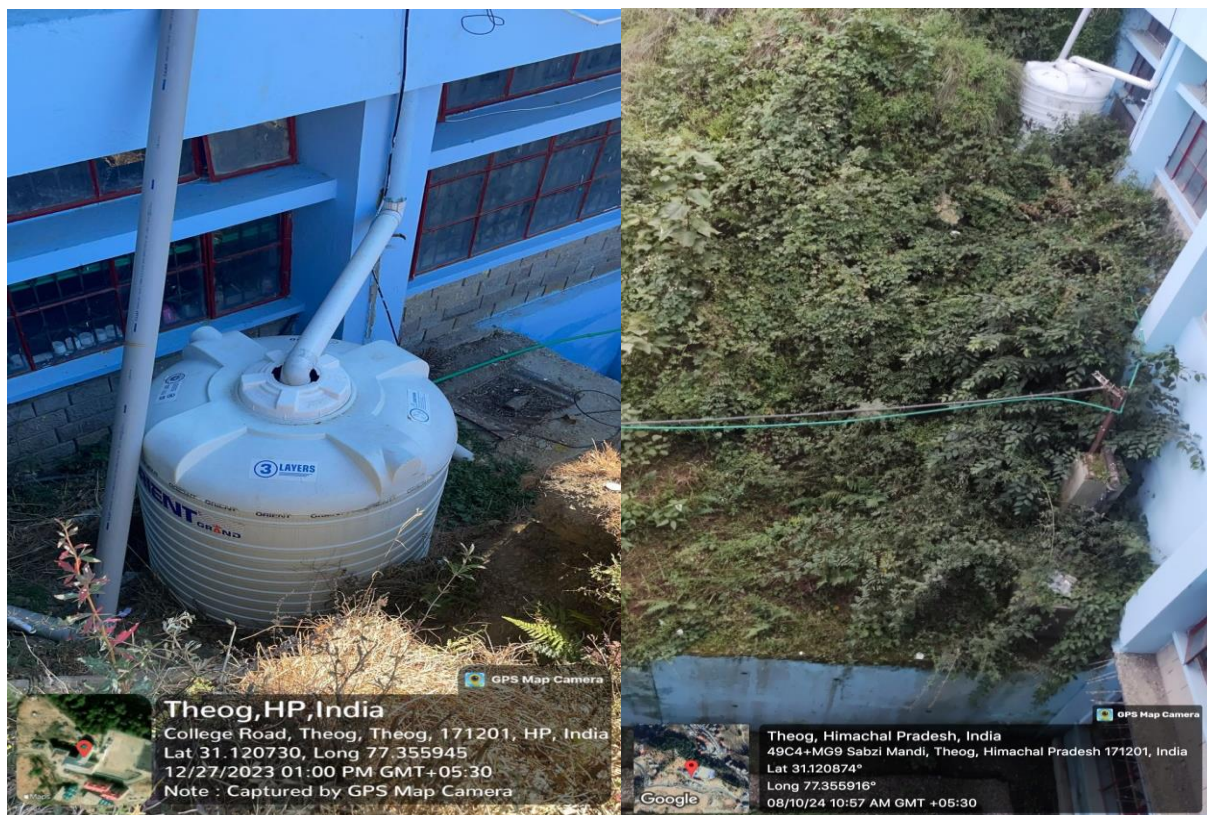
Rainwater harvesting Tank and its connectivity to Botanical glass house and Toilet
